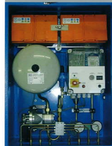
Power supply with battery pack
